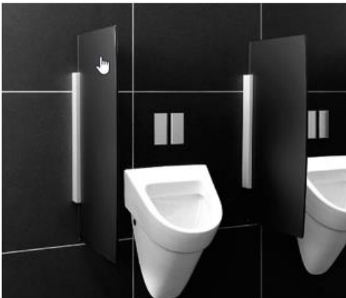
Automatic flushing (IR-detective)
